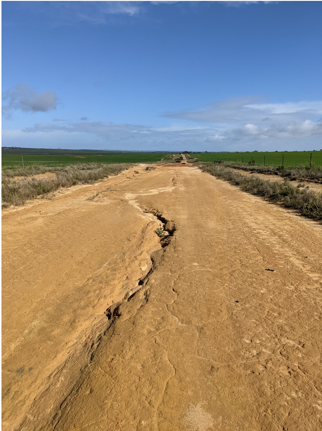
Figure 1. An example of the erosion on the eastern end of the existing track (looking west)
